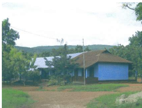
Aseseeso JHS with a part of the roof still to be completed, and freshly painted walls, July 2008
