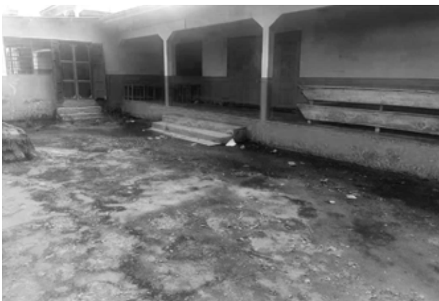
Flooding damage at Hartley Trust School
